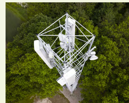
Mast in Denmark
