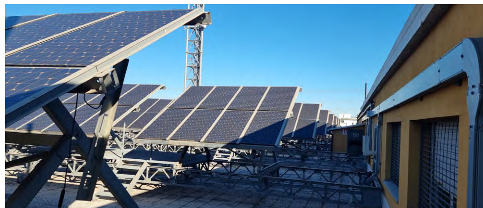
Wind Tre solar panels
