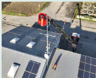
Drei Wetter meteorological sensor on a building
