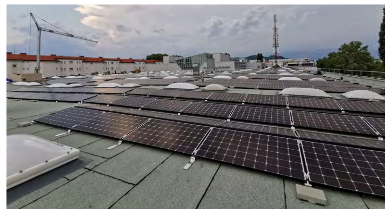
Rooftop solar in Austria
